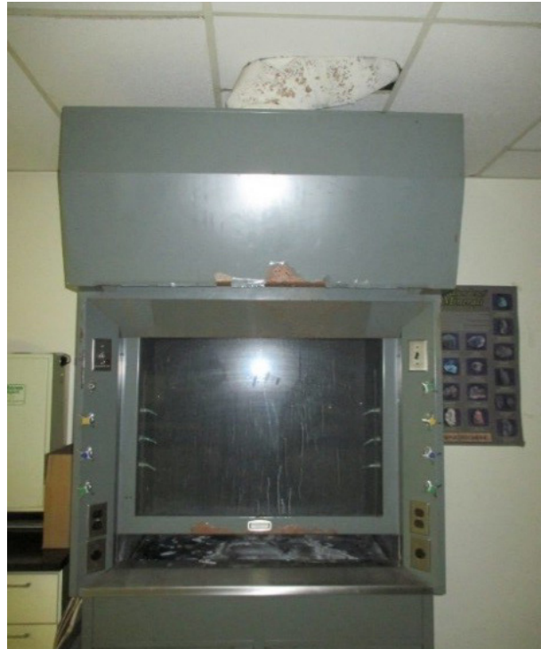
Mechanical Photograph #10 Chemical Fume Hood
