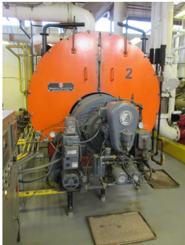
Mechanical Photograph #1B Main School Boiler
