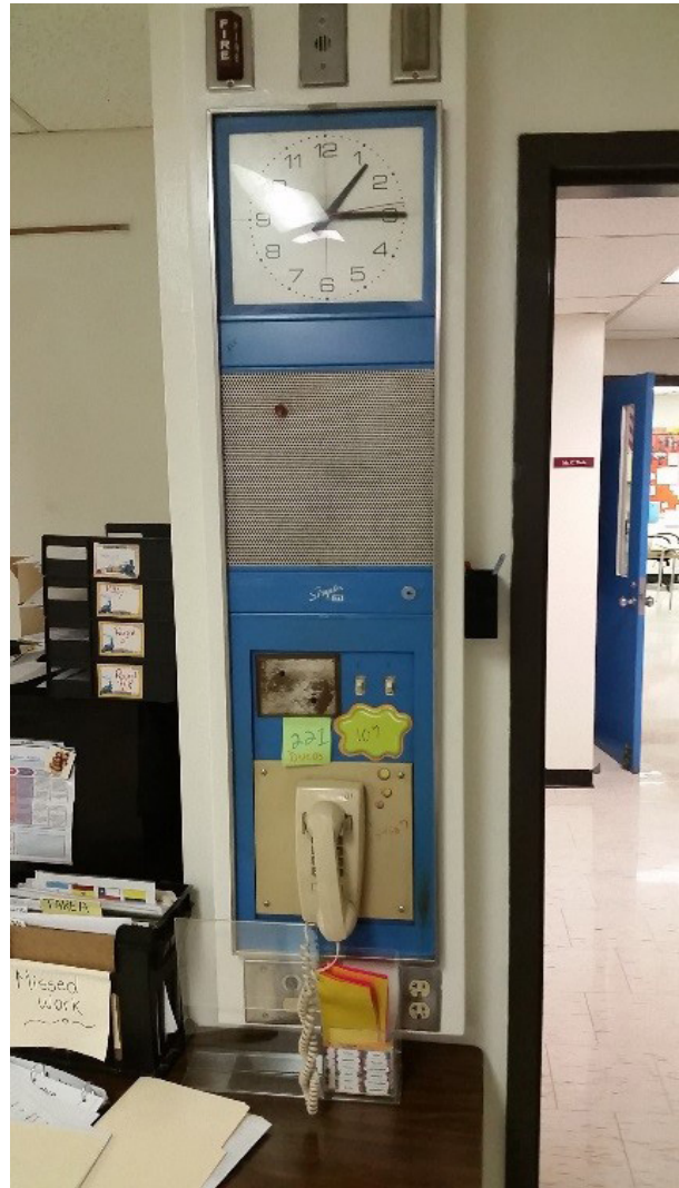
Electrical Photograph #14 Classroom Utility Panel
