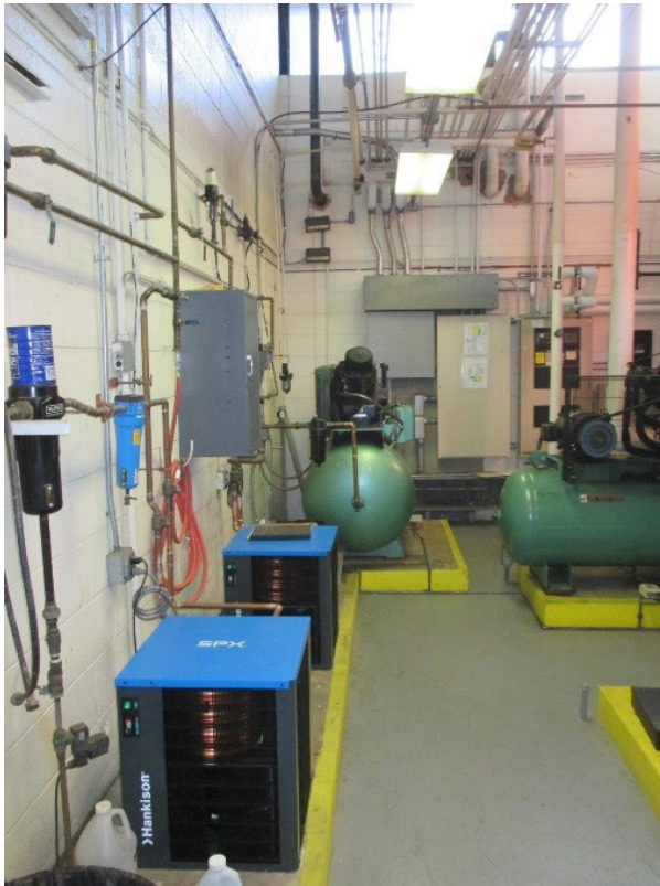
Mechanical Photograph #15 Existing Air Compressors
