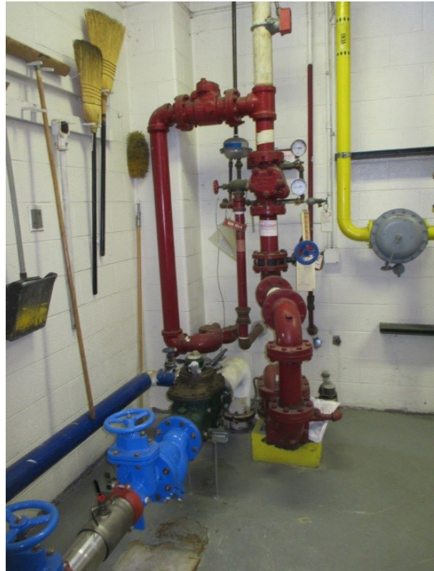
Mechanical Photograph #11 Wet Pipe Riser in Main Mechanical Room
