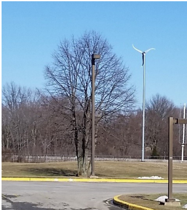
Electrical Photograph #12 Exterior Lighting Fixtures - Parking Lot
