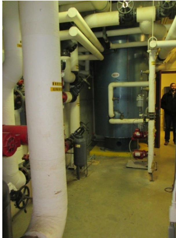
Mechanical Photograph #13 Domestic Water Storage Tank
