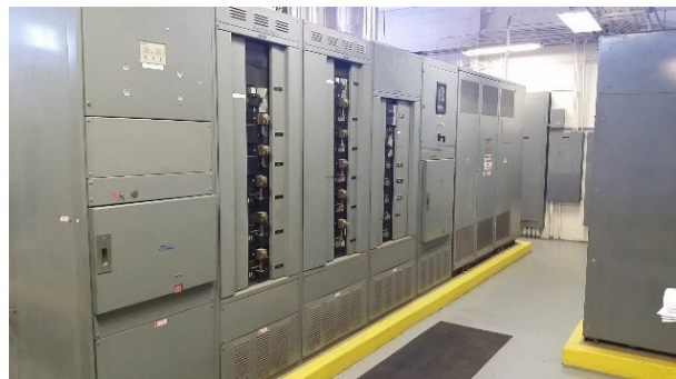
Electrical Photograph #2 2000kVA Transformer and Switchboard
