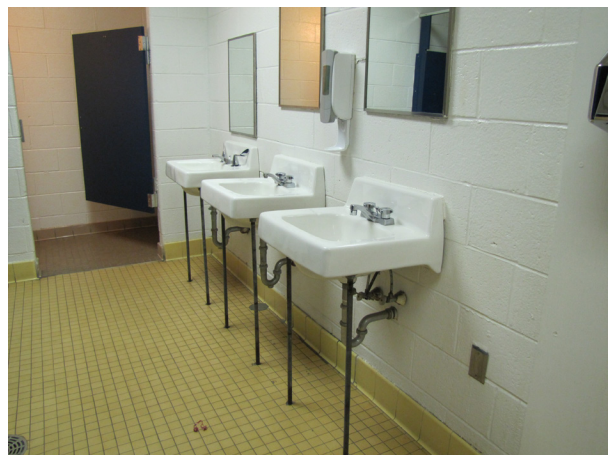
Figure 1.4 Non-Code Compliant Issues Throughout
