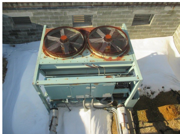
Photograph #4 Air Cooled Chiller
