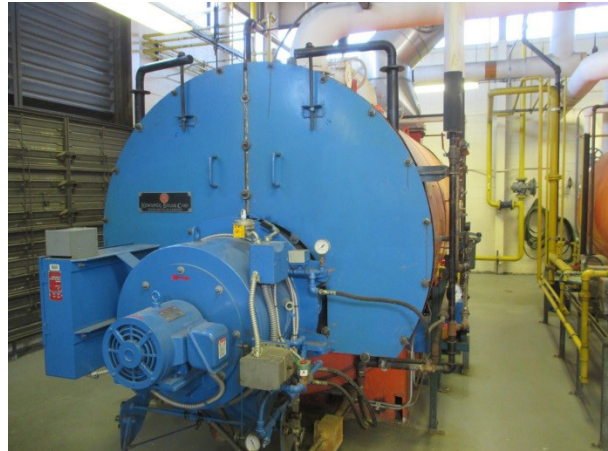
Mechanical Photograph #1A Main School Boiler
