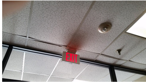
Electrical Photograph #18 Upgraded Addressable Devices
