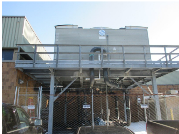
Mechanical Photograph #3 Cooling Tower
