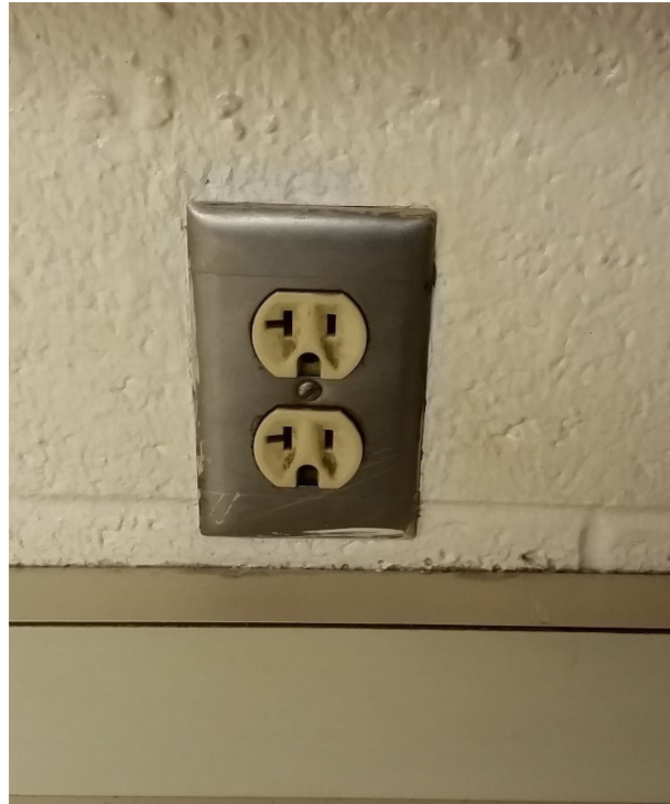
Electrical Photograph #5 Typical Receptacle
