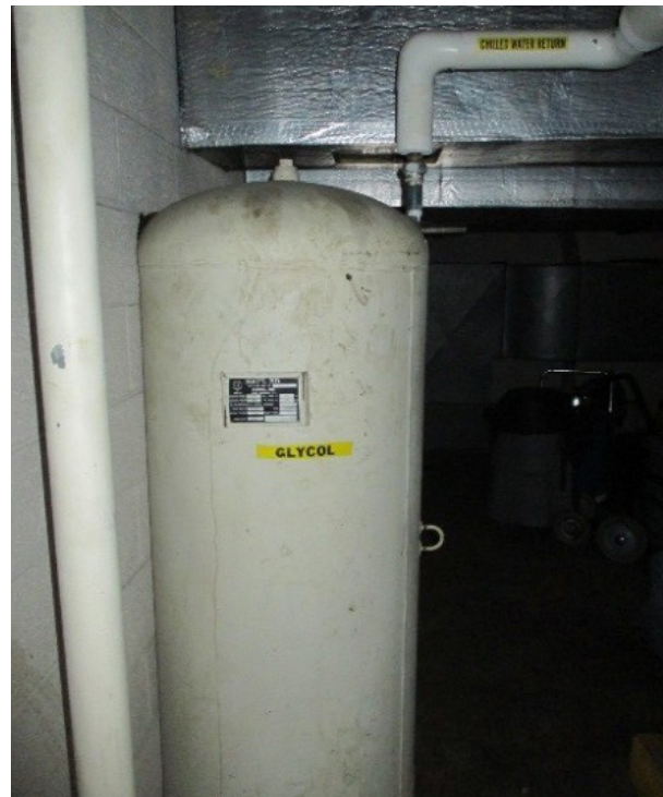
Mechanical Photograph #9 Kitchen Make-up Air Unit Glycol Expansion Tank
