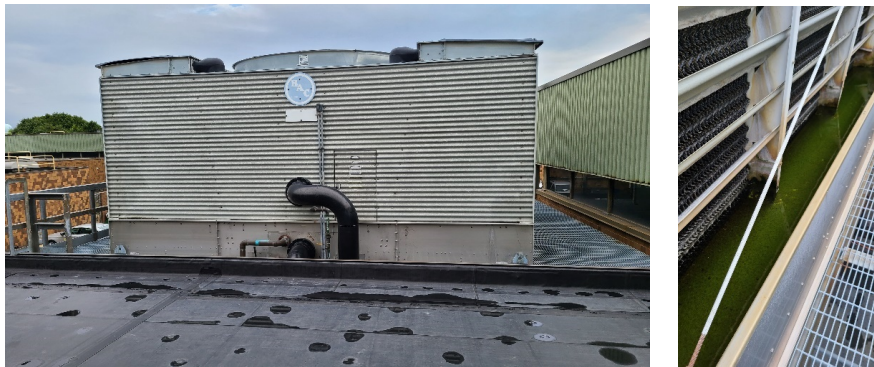
Figure 2: Cooling Tower and Basin (showing green water)
