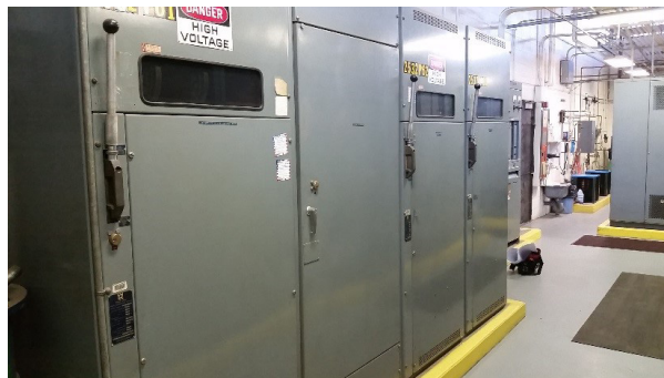
Electrical Photograph #4 Kohler Generator
