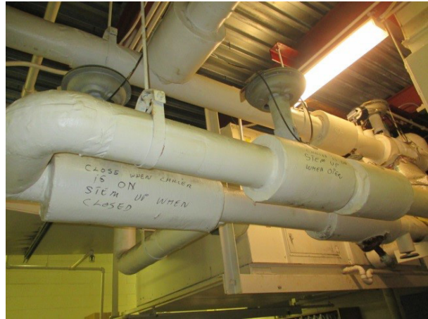
Photograph #5 Air Cooled Chiller Changeover Valves
