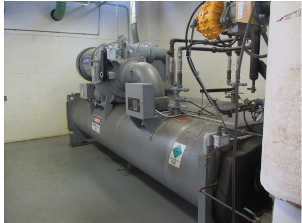
Mechanical Photograph #2 Water Cooled Chiller
