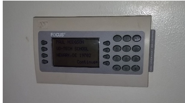
Electrical Photograph #21 ADT Security System Control Panel
