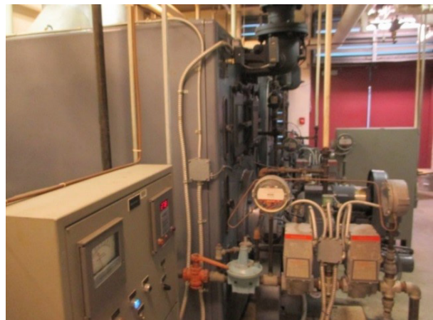
Mechanical Photograph #7 Gym Hot Water Boilers
