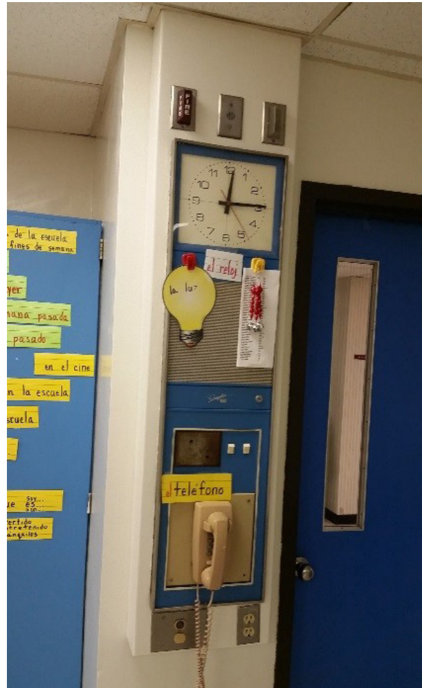
Electrical Photograph #19 Classroom Utility Panel with Non-Addressable Devices
