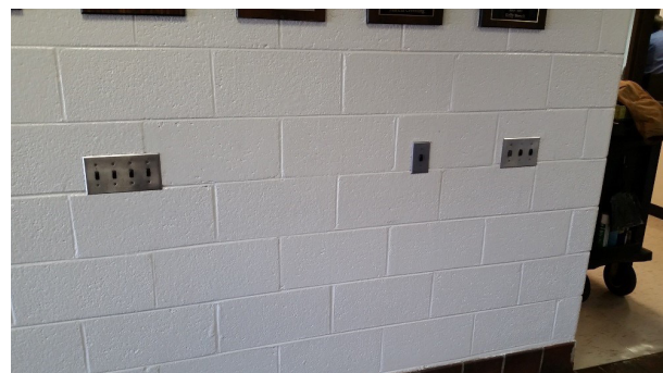
Electrical Photograph #15 Existing Keyed Lighting Switches
