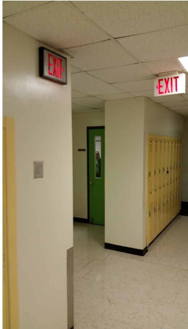
Electrical Photograph #16 Mis-Matched Exit Signs
