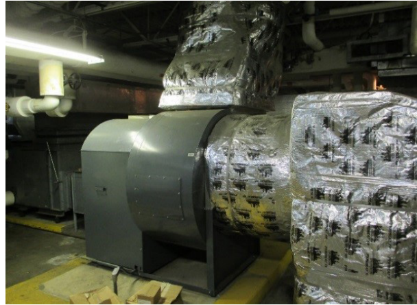
Mechanical Photograph #8 Kitchen Hood Exhaust Fan
