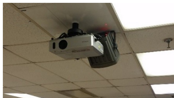
Electrical Photograph #25 Overhead Projector and Speaker
