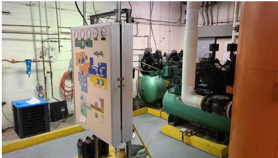
Figure 5: Pneumatic Controls Compressors, Dryers and Representative Panel
