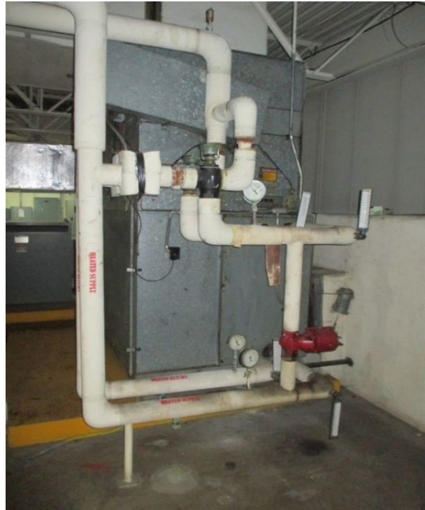
Mechanical Photograph #6 Typical Air Handling Units
