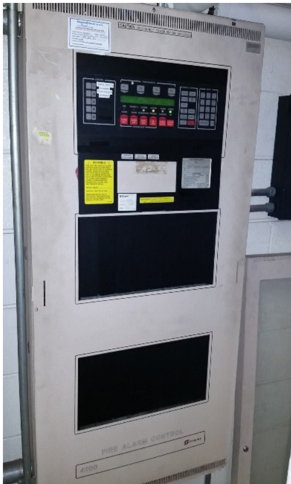
Electrical Photograph #17 Simplex Grinnell Fire Alarm Control Panel
