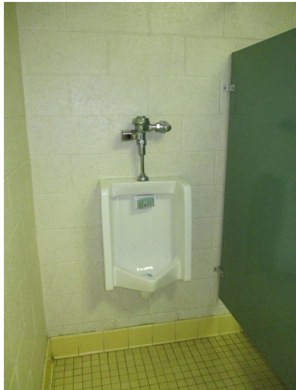
Mechanical Photograph #12 Typical Urinal
