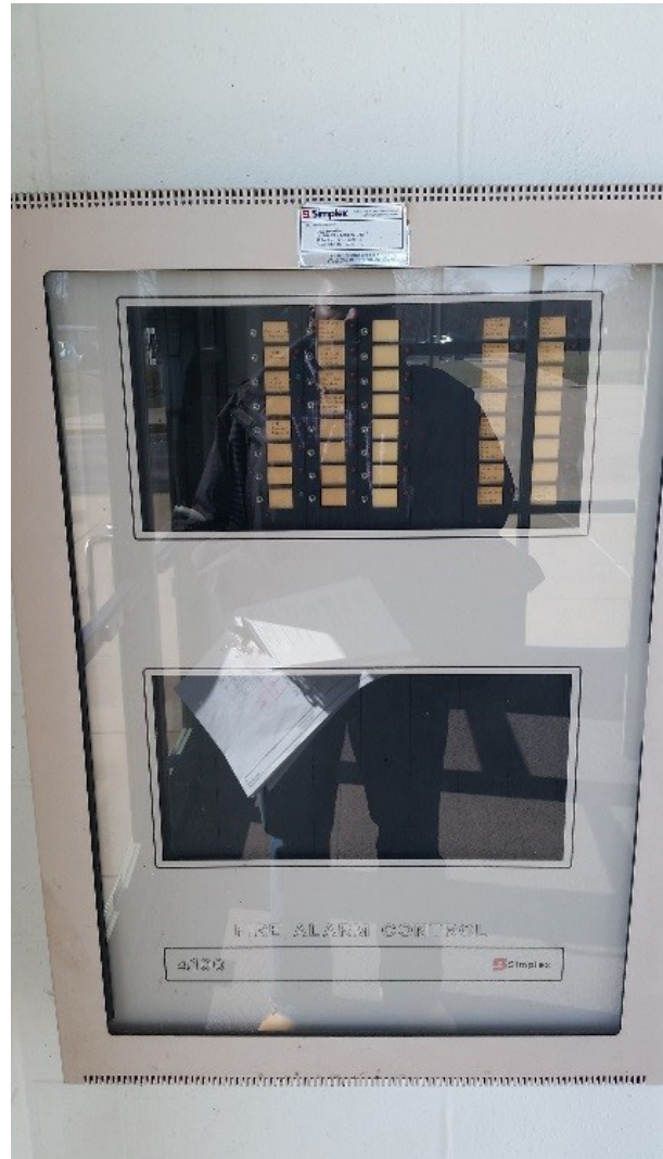
Electrical Photograph #20 Simplex Grinnell Model 4100 Fire Alarm Control Panel with Voice Evacuation
