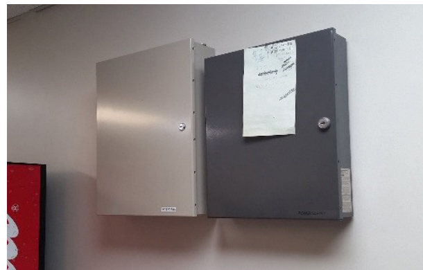
Electrical Photograph #22 ADT Security System Power Supply Panels
