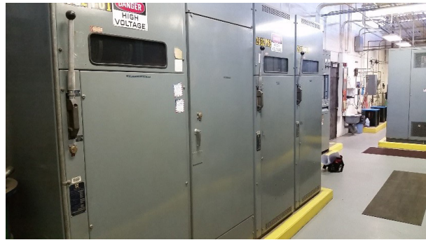
Electrical Photograph #1 Incoming Primary Metering Compartment and Primary Switches
