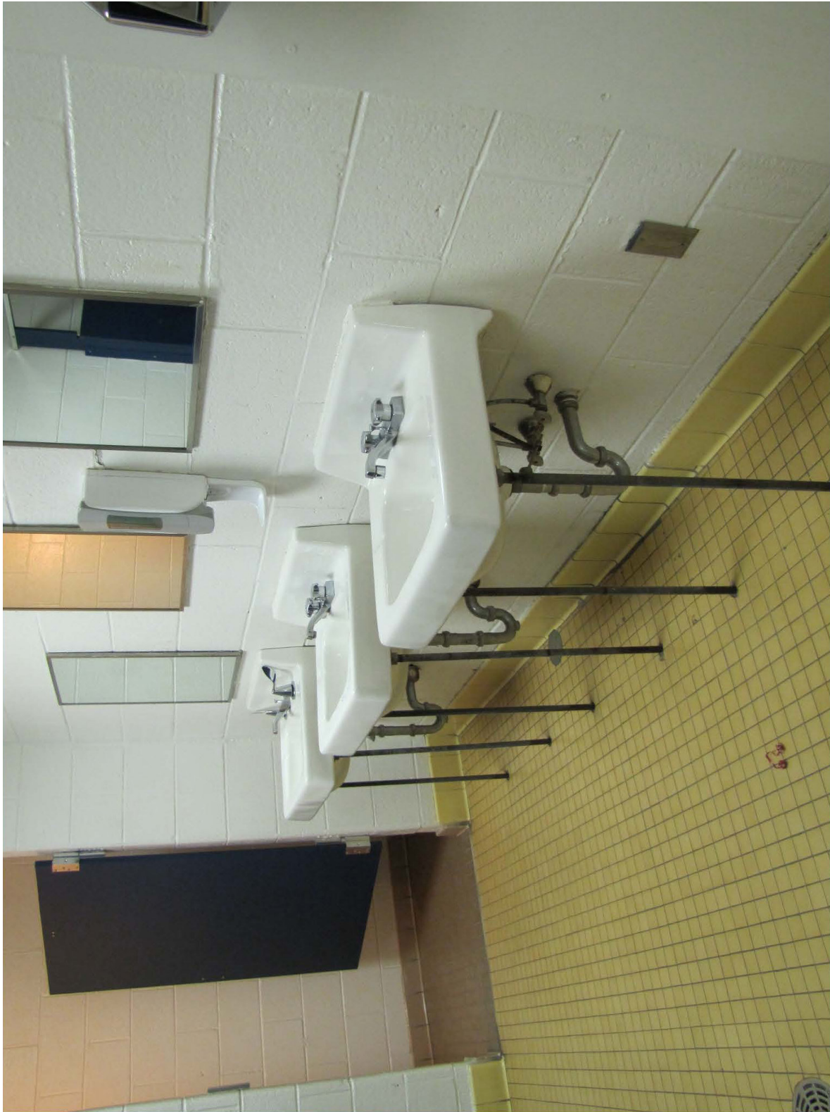
Figure 1.4 Non-Code-Compliant Issues Throughout
