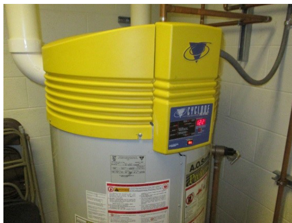
Mechanical Photograph #14 Domestic Hot Water Heater
