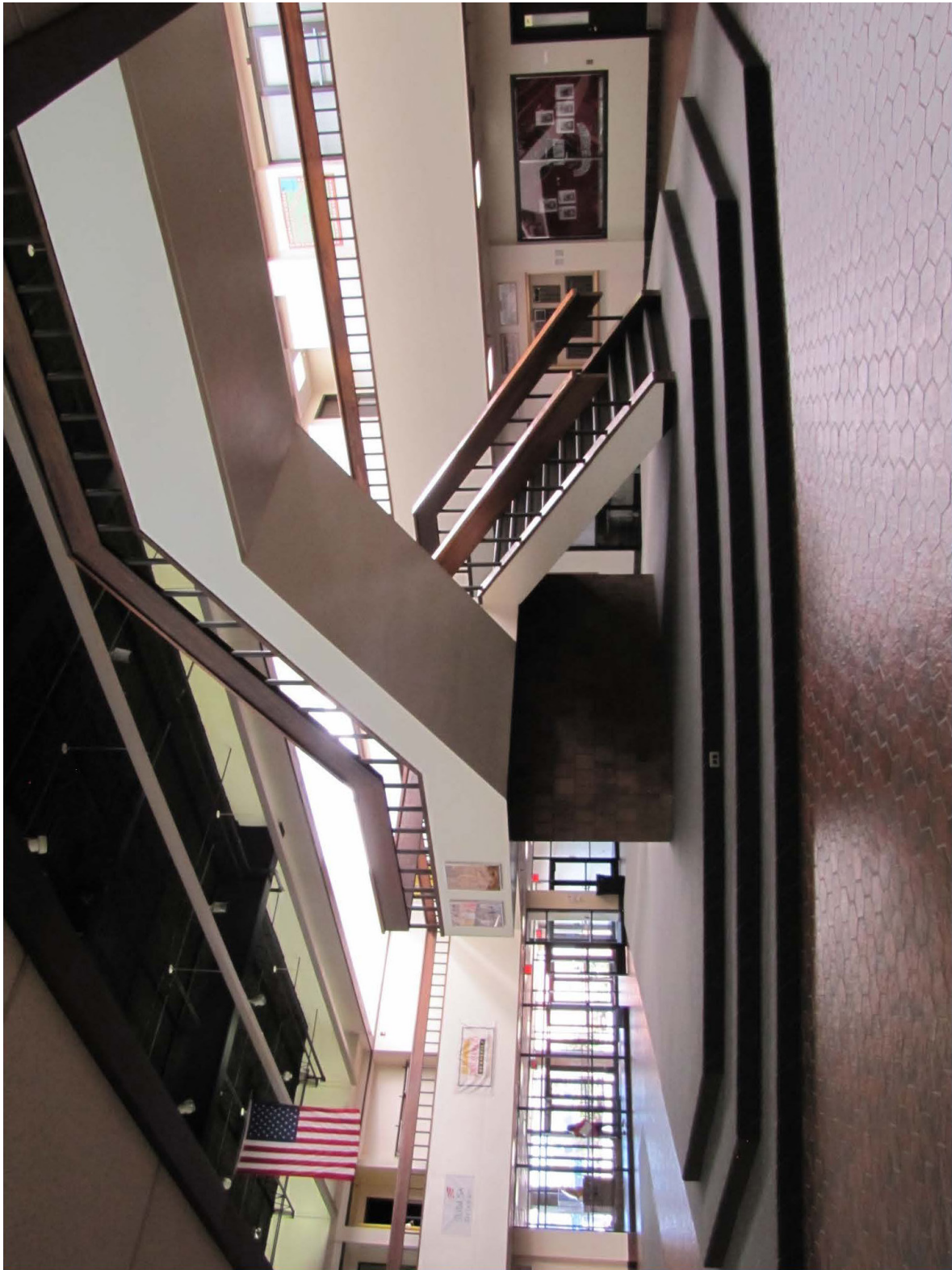
Figure 1.3 Non-Code-Compliant Issues Throughout
