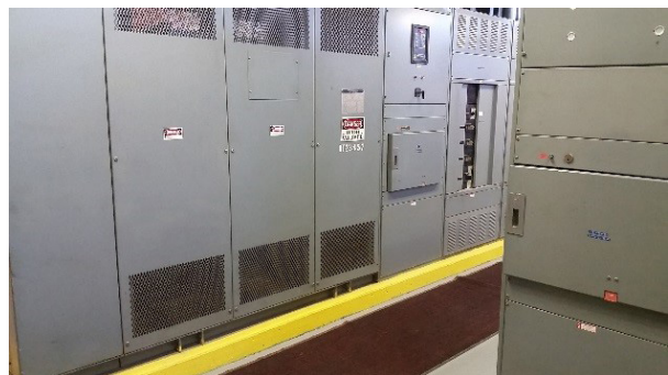
Electrical Photograph #3 1500kVA Transformer and Switchboard
