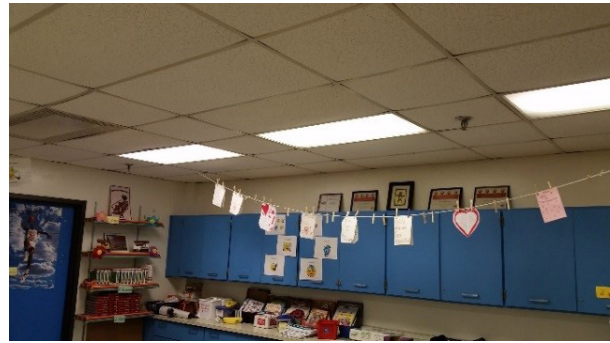
Electrical Photograph #7 Typical 2'x4' Acrylic Lens Fluorescent Fixtures
