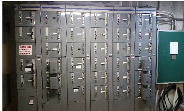
Electrical Photograph #6 Typical Motor Control Center
