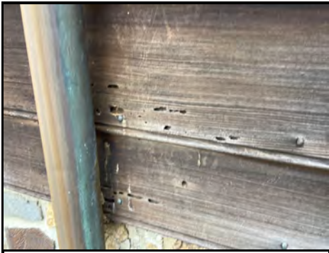
Carpenter bee damage
