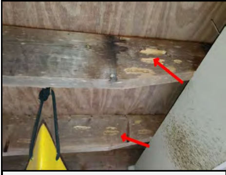
Carpenter Bee Damage
