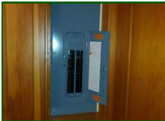
Location: STUDIO GARAGE
