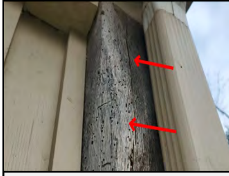
Wood boring beetle damage
