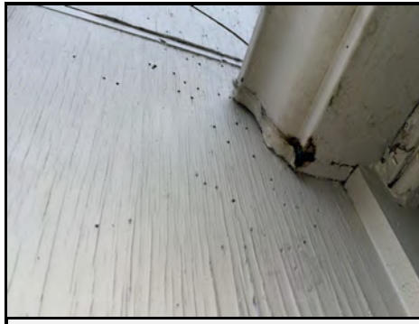
Powder post beetle damage
