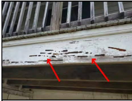
Carpenter Bee Damage
