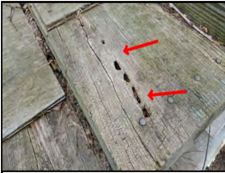
Carpenter Bee Damage
