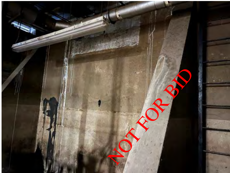
Southeast corner of the tank vault detail with the sidewalk vent to the left.
