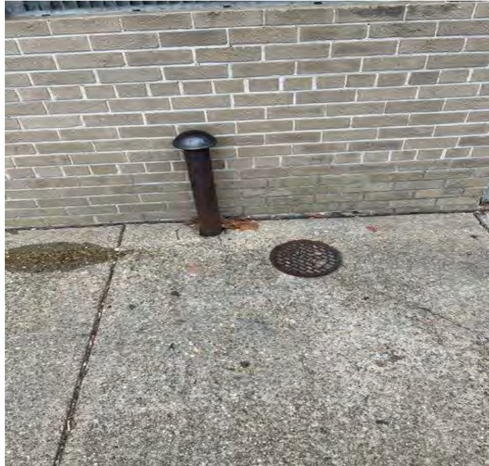
The Fill and the vent pipe located to the south of the tank below Room 114 windows.
