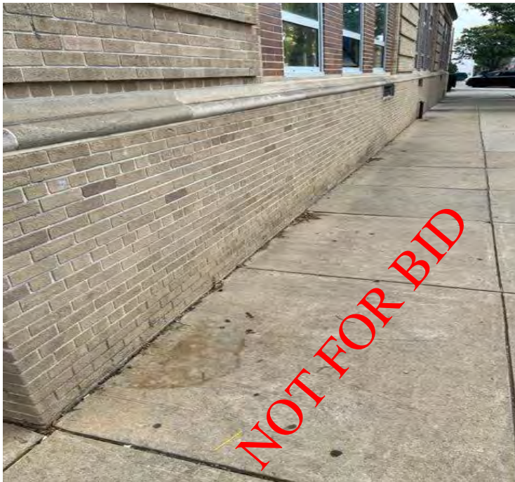
Looking from the southwest corner of the building towards the tank fill and vent approximately 65 feet to the east below Rm 114 windows.
