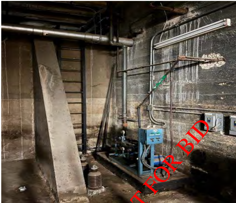
Access ladder and heating oil pump indicated. Green line is the supply line to the boilers.
