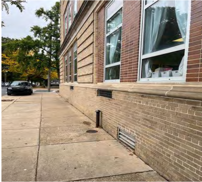
The tank fill and vent located along the 7 th St sidewalk with Lombard St in the distance. The louvered vent indicated is located above the southeast corner of the tank vault, in the transformer room.
