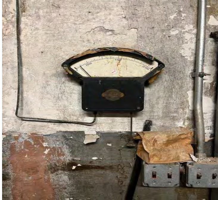
Tank gauge indicating 800 gallons of heating oil.
