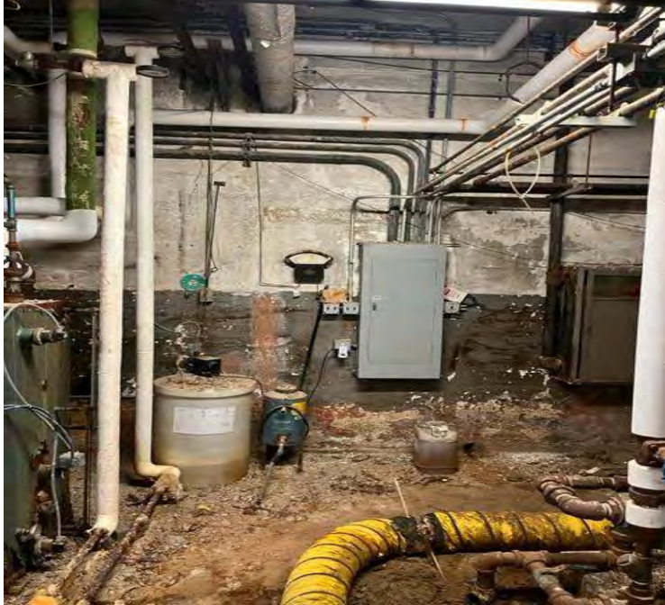
Gauge indicated. Tank is located behind the south boiler room wall (indicated) to the right of the gauge.
