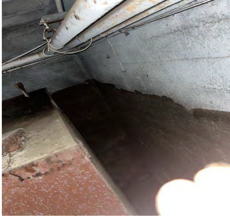
South end of tank indicated. Tank is separated from surrounding walls by approximately 2 feet each way. Tank is believed to rest on the basement slab.
