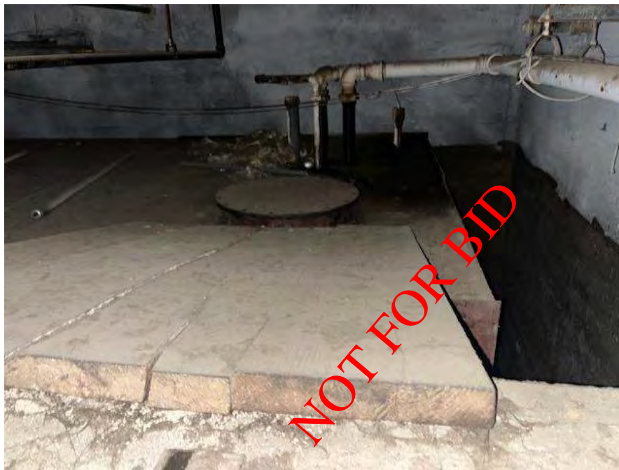
Manway at north end of tank. Supply and return lines are indicated.
