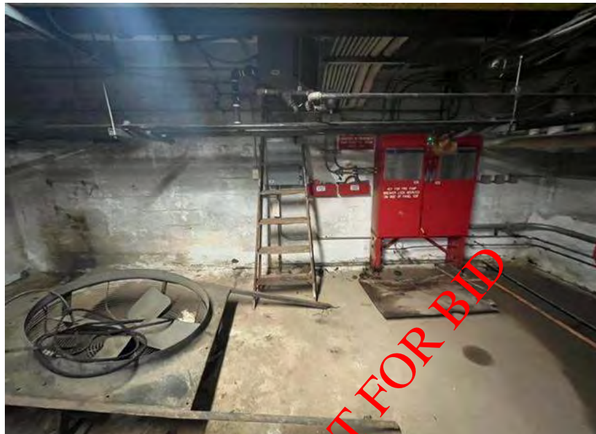
Storage Room south wall, adjacent to north side of tank vault, (shared wall). Floor indicated is approximately 4' above boiler room/ transformer room elevation.
