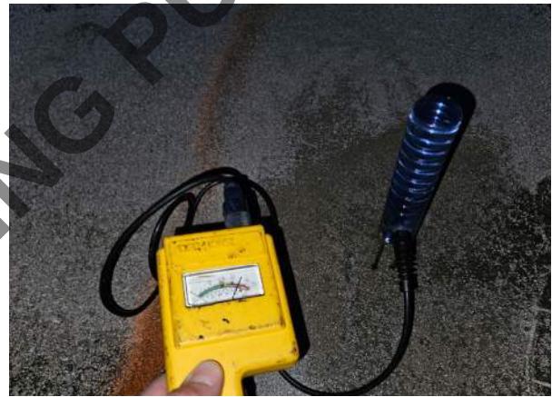
Probe #03 Confirmed Wet
