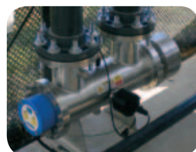
UV Disinfection System
