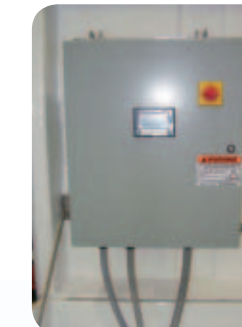
U.L. Listed Control Panel
